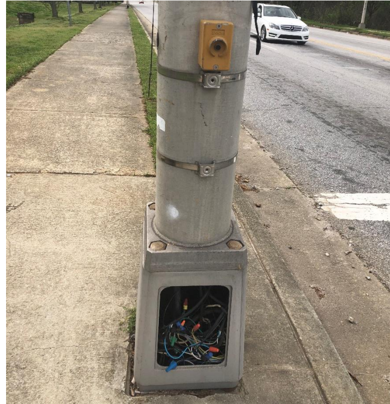
Figure 15. Broken walking light signal in Mechanicsville
