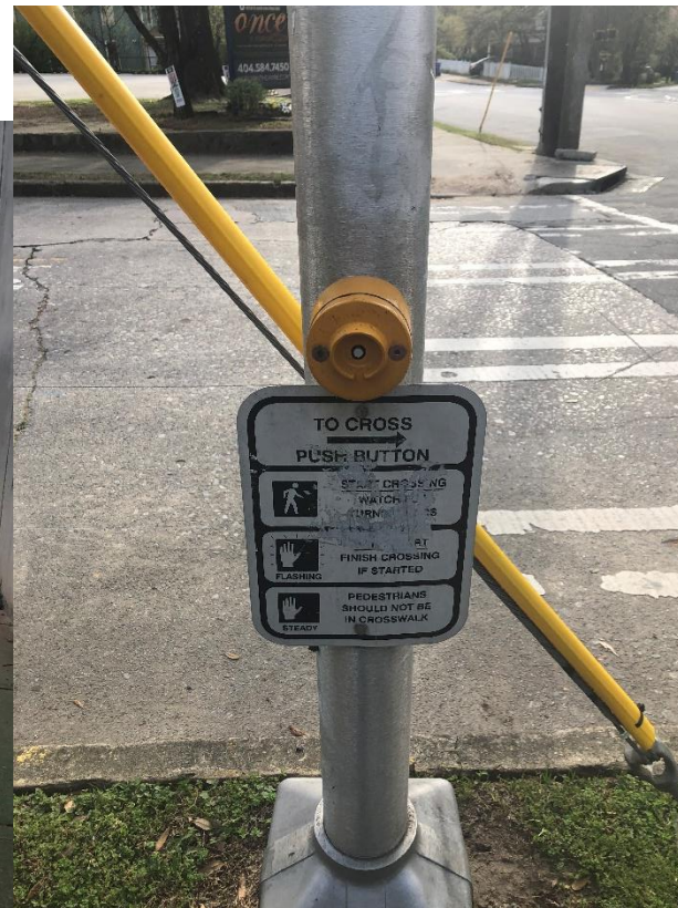
Figure 24. Broken pedestrian walk signal near Inman Park
