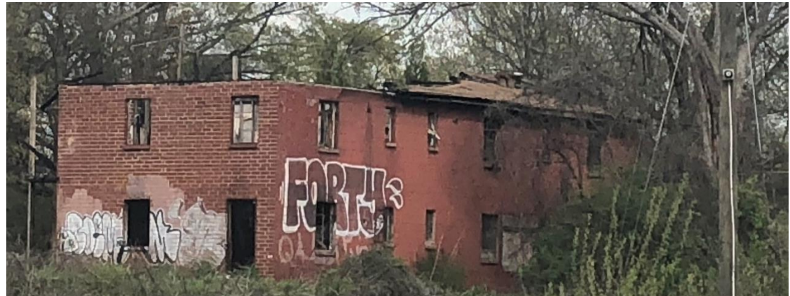
Figure 11. Abandoned building in Mechanicsville
