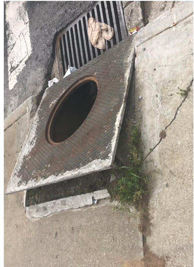
Figure 40. Lifted sidewalk in Mechanicsville
