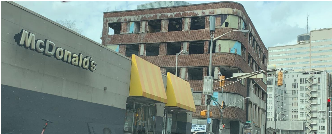
Figure 12. Abandoned building next to McDonald's restaurant near Mechanicsville
