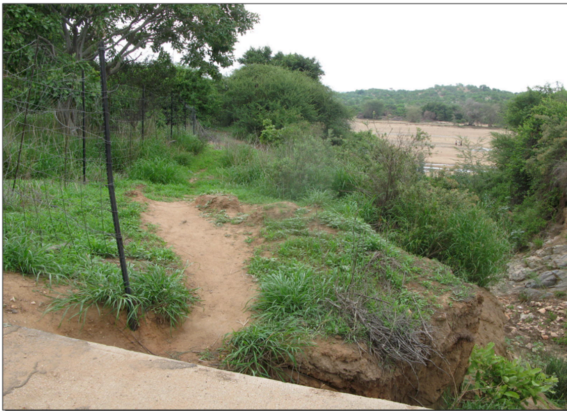
Fig 8: An undesigned crossing point showing a portion of the vandalized fence. [Courtesy of T. Muleya]
