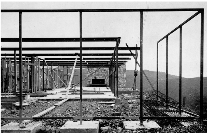
Figure 14: Photograph of Case Study House #16’s steel frame and stone fireplace. Craig Ellwood, “The New Case Study House,” Arts and Architecture , December 1952, 22.
