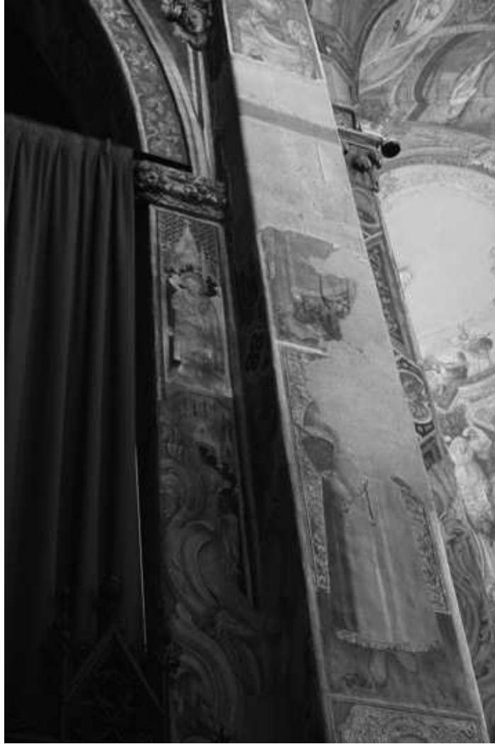
Figure 28. Detail view of right pilaster of the left apse chapel (Teodelinda Chapel), wall painting, Basilica of San Giovanni, Monza. (Photo by Author)
