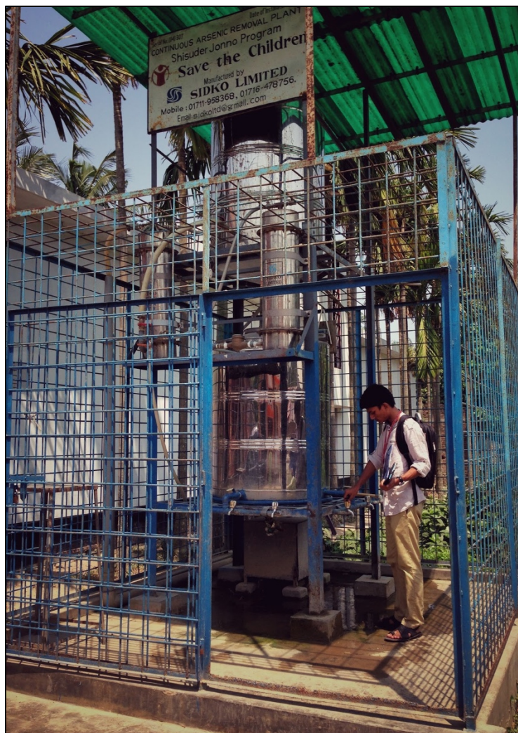
Figure 4. One of SC's WTPs in Meherpur (Photo credit: Anushree Y. Mahajan).
