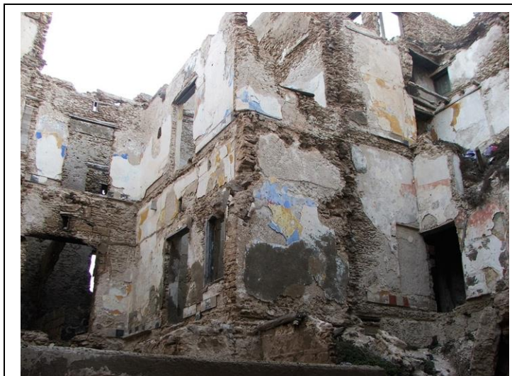
Figure 11 The rubble of a partially-demolished house in Essaouira
