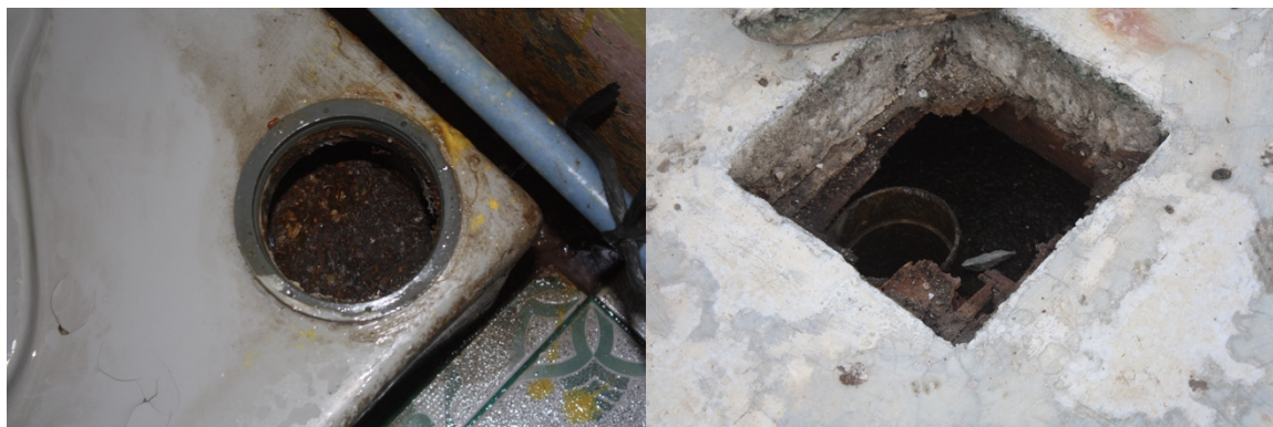
Figure 8. Fecal Sludge Accumulation Access
