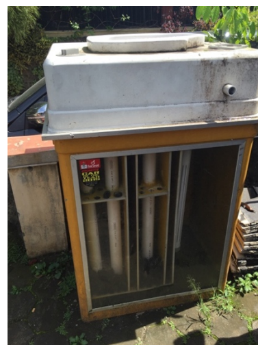
Figure 14. Sanitation System Type 3 (No filter media)
