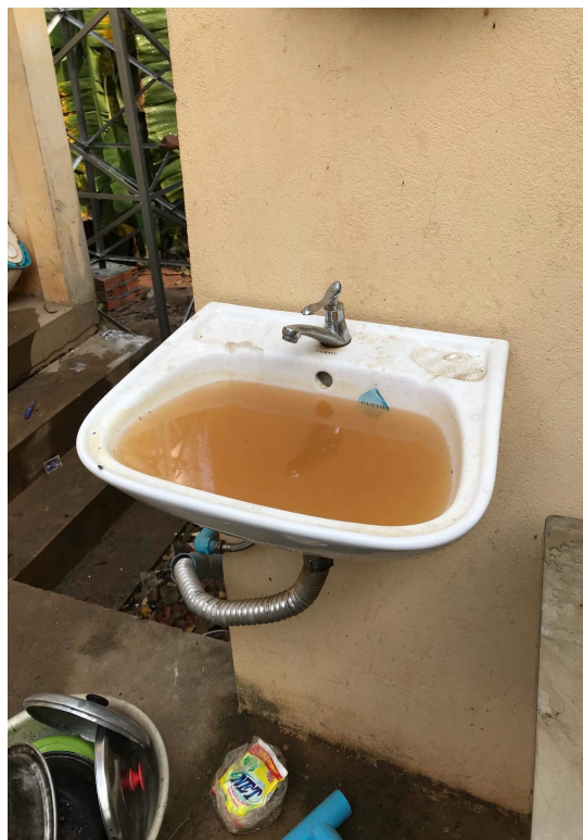
Figure 2. A sink in health center B
