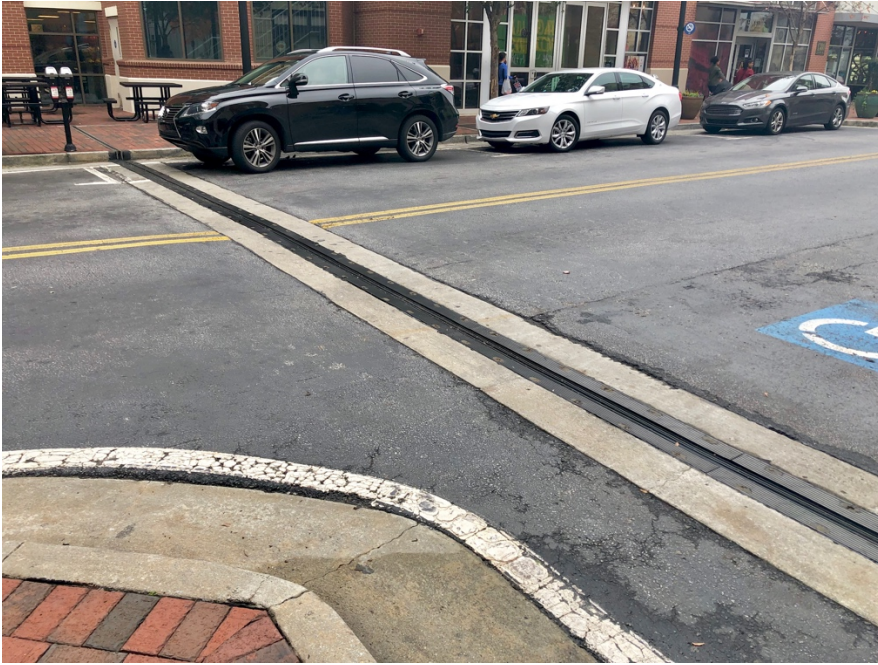
Figure 19. A larger expansion joint, crossing Atlantic Drive, spans across the road and adjacent sidewalks.
