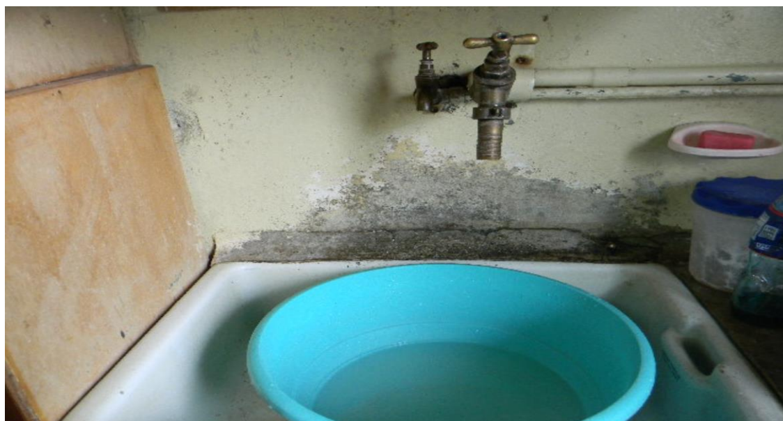
Figure 16: Sink taps within the hospital.
