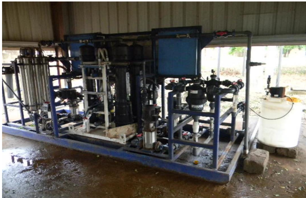
Figure 3: GE donated Homespring, amiad, and membrane filter, with chlorine doser
