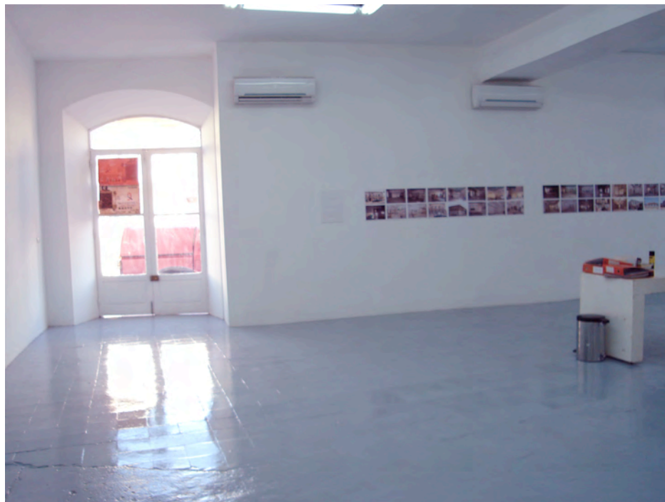
Fig. 12. Section of Unap building before and after renovation for a gallery space for the Trienal de Luanda. The rest of the building is in bad repair, with major structural problems.
