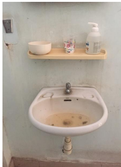
Pictured above: A sink located outside a conference room where hospital staff occasionally discuss cases. This sink area is located directly around the corner from the delivery room. Pictured are a bottle of hand sanitizer and a cup of detergent on the shelf above the sink.
