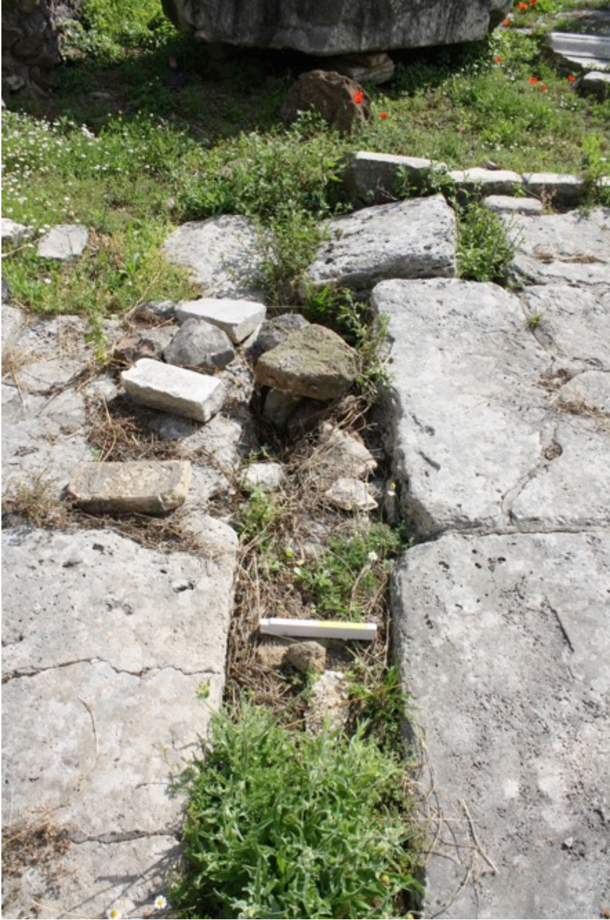
Figure 17. Drainage channel, Appiades Fountain (Phase I, Caesarian period). Photo: Beth Gardiner Lytle.
