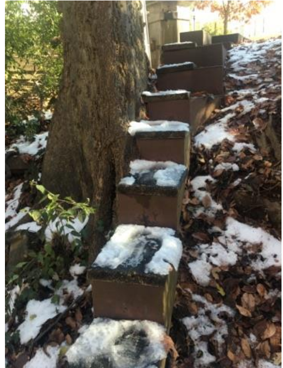
Figure 14. Wood and steel steps at the top of the southern slope. Personal photograph by author.
