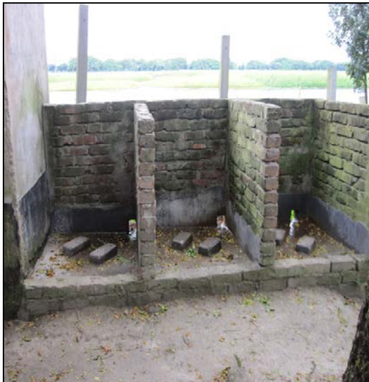
Figure 4.3 Open School Urinal
