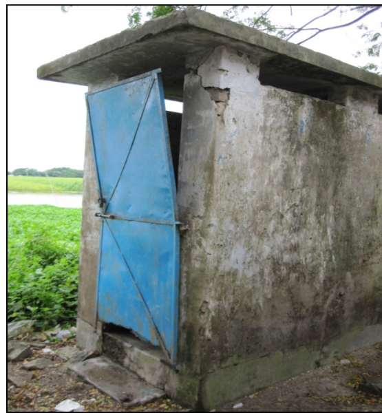
Figure 1.2 Broken and abandoned school latrine
